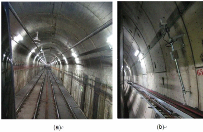
Fig. 2. (a) Photo of classical arched tunnel used in measurements. (b) Photo of transmitter fixed inside tunnels.
