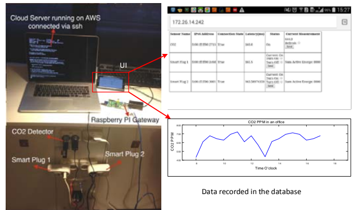
Fig. 2. Implemented hardware of the minimal system including the Cloud Server, User Interface, Automation Gateway, and the WSAN devices, and the CO2 measurements collected over a normal working day in the office building
