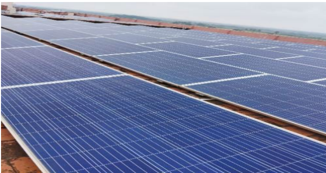
Figure 7. 33 kW solar PV system used for data collection
