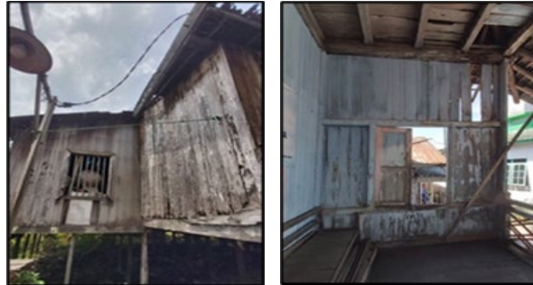
Fig. 3. The Exterior Walls of the House Showing Signs of Rotting and Damage (Author, 2023)
