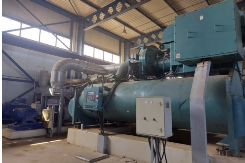
Fig. 2. Photo of the Real System (Chiller 1) in Basra International Airport.
