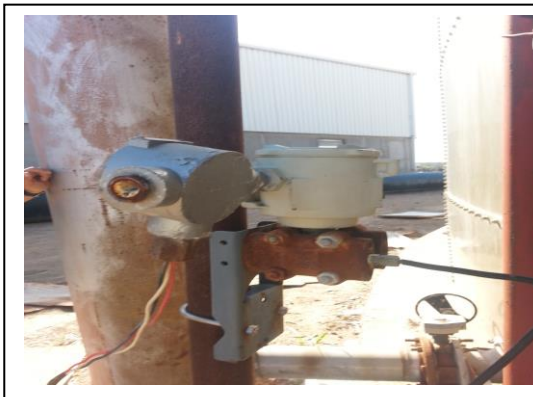
Fig 14. level transmitter (LT-604) in the water treatment unit.
