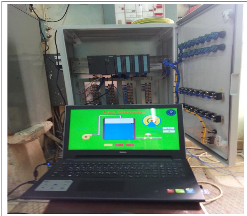
Fig 23. Photograph of overall measurement and monitoring system.
