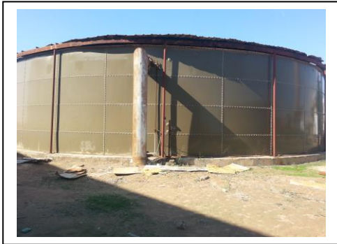
Fig 12. water vessel (V-604) in the water treatment unit.
