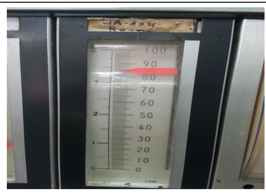
Fig 15. level indicator (LI-604) in the water treatment unit.
