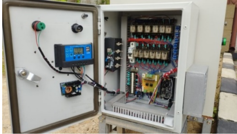
Figure 7. Solar charge control
