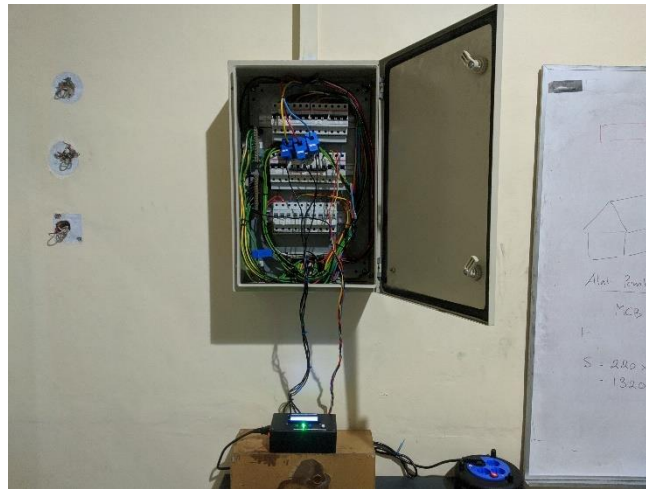
Fig. 10. The implementation of a data logging monitoring system
