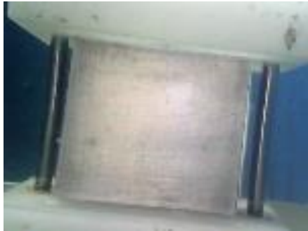
Fig 3. Front View Before Corrosion
