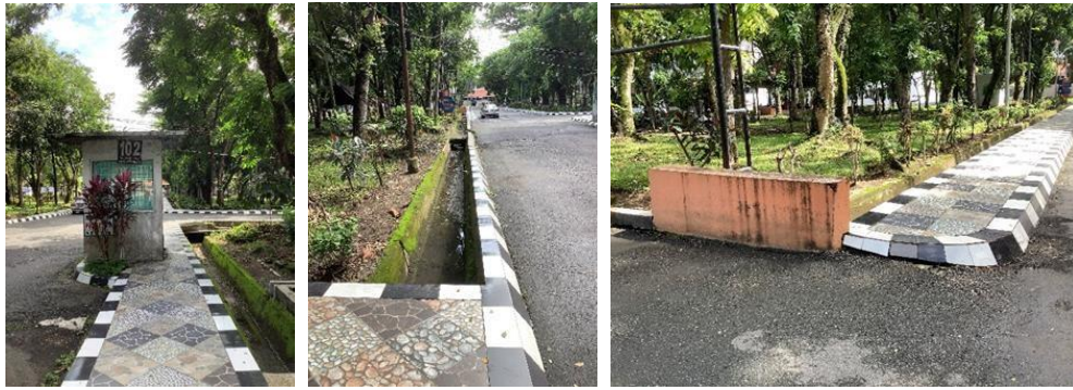
Fig. 6. The platform conditions do not follow design standards requirements.
