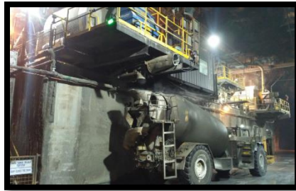
Fig. 1. Loading Point Shotcrete Material from the Batch Plant to the SVS Truck
