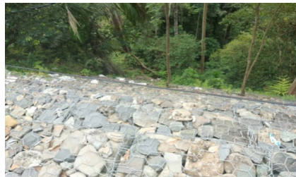
Figure 4. Landslide Mitigation Efforts at Way Krui
