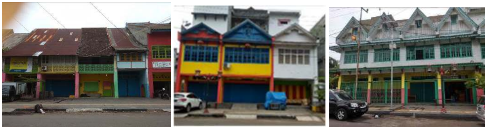
Fig. 6. (a) Zinc roof ; (b) Rolling doors ; (c) glass windows with timber frame
