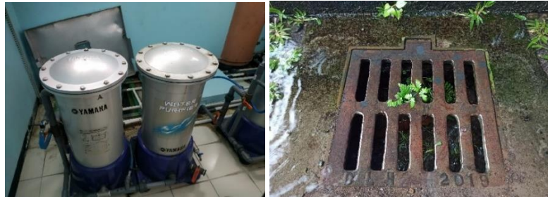
Fig. 2. Drinking Water Filtration and Infiltration Wells
