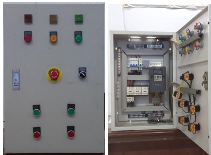
Fig. 4. Programmable Logic Controller Panel
