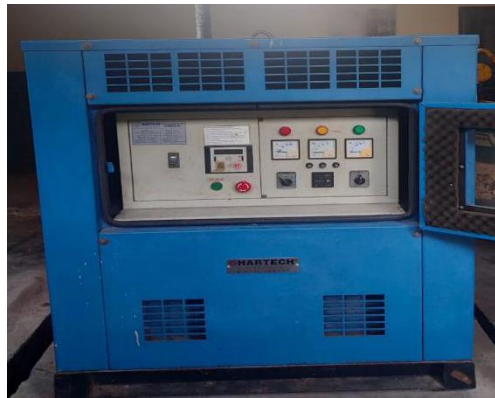
Fig. 2. Generator set on RRI Tarakan City.
