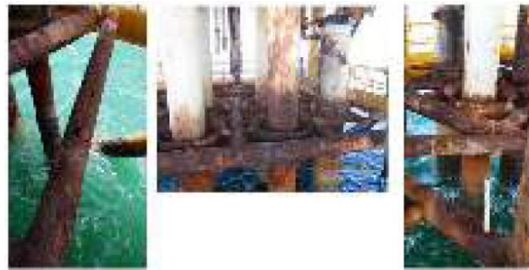
Fig 2. An example of the conditions of aging offshore platforms in Indonesia [2]
