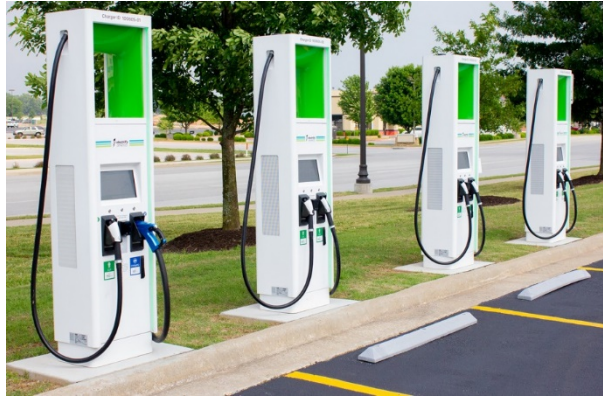
Figure 4 Example of EV public charging station in America [30]
