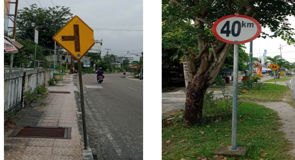
Fig. 1. Good-condition signs and damaged-condition signs
