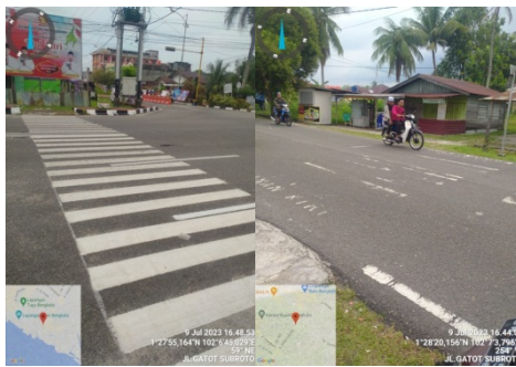
Fig. 2. Good condition markings and bad condition markings
