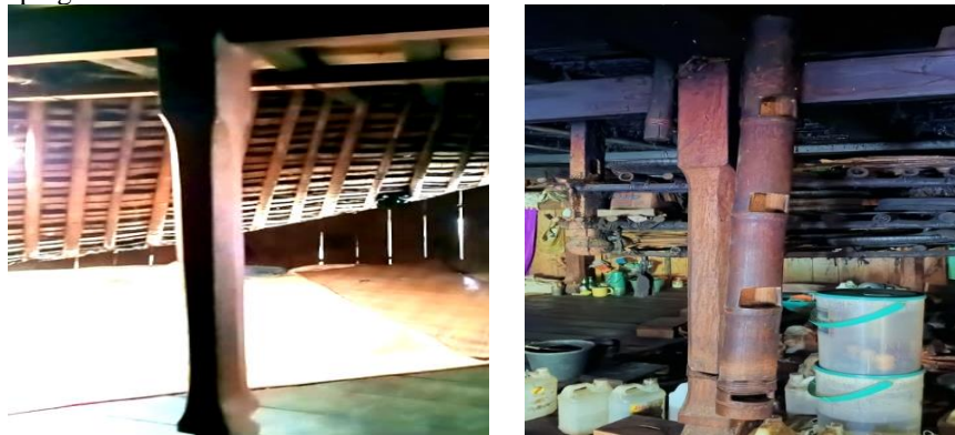
Figure 2. The pillars of the Mbaru Niang and Siri Bongkok traditional houses (middle pillar)
