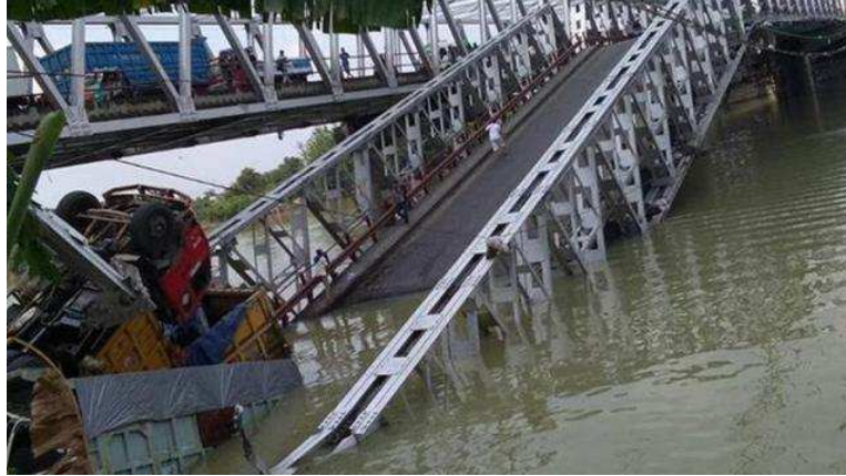
Fig. 2. The Collapse of Cincin Lama Bridge Source: Suara Merdeka Newspaper
