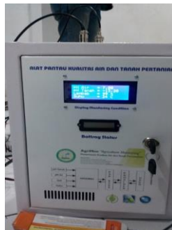
Fig. 1. The Control Panel
