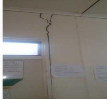
Fig. 3. Vertical crack on another building
