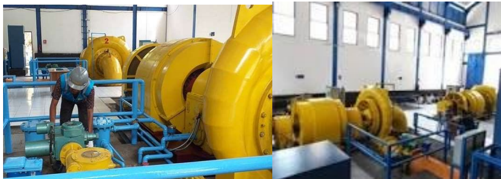
Figure 5. Ndungga Ende PLTM Turbine and Generator (Sindonews.com, 2019)
