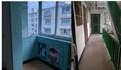
Figure 4 Left: Single-layer FRP windows on the balcony right: old house corridor and iron fence door
