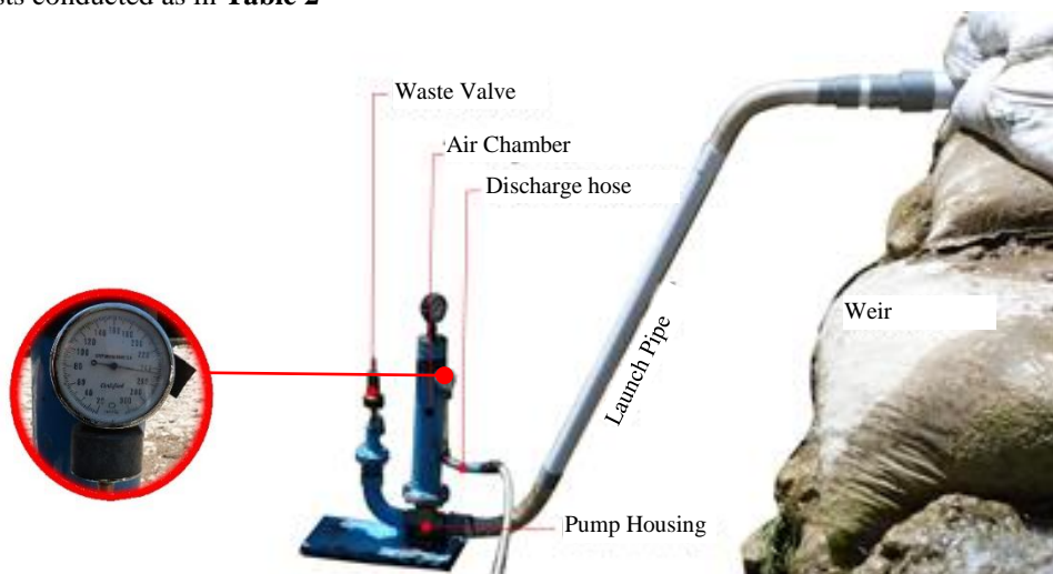
Figure 4. 1½ inch ram pump installation
