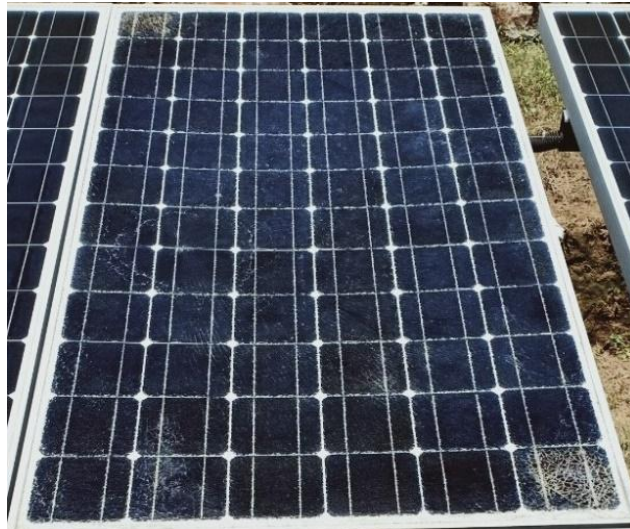
Figure 4. Microcracks of a PV module at Hoineno system
