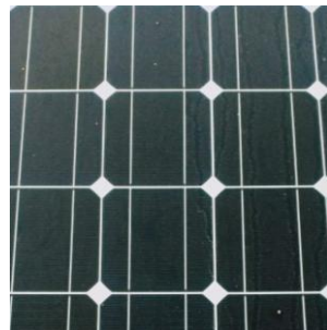
Figure 2. Discoloration of PV modules at Hoineno
