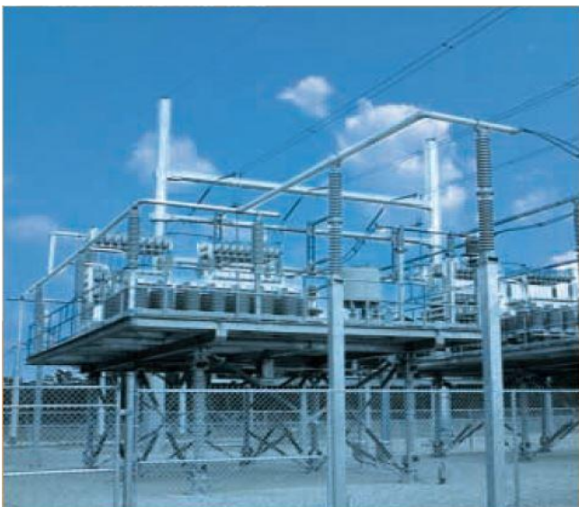
Figure 1. Series Capacitor compensation (70%) in the USA.
