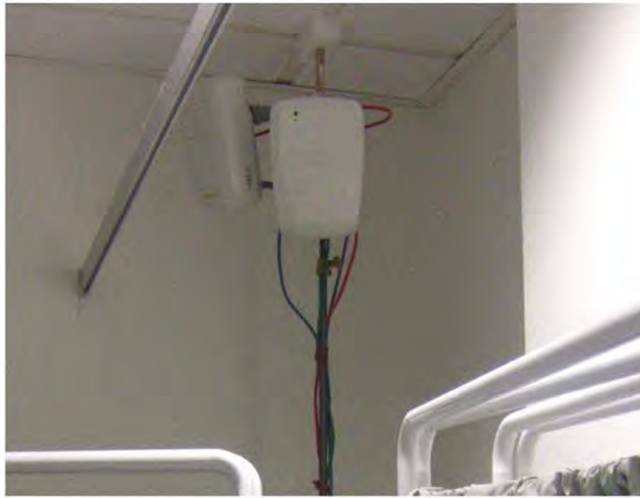
Fig. 4. Ubisense sensors installed in the ward.
