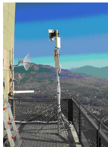
Figure 5. Pre-WiMAX outdoor installation
