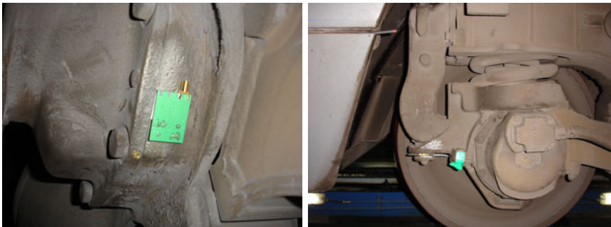
Fig. 5. SAW Temperature Sensor and Antenna Installation for Axle Box Bearing Temperature Measurement
