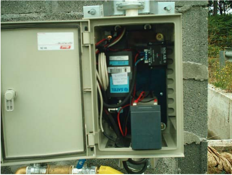
Fig. 3. EZS data acquisition and communications system assembled in the protection box
