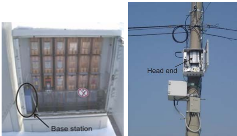
Fig. 4. Example of practical placement of base station (i.e. head end) in on-the-ground transformer station (left – Source: Drewag, Dresden, Germany) and on a pole near to the aerial transformer; example from Asia (right - Source: Kepco, Jeju Island, South Korea)
