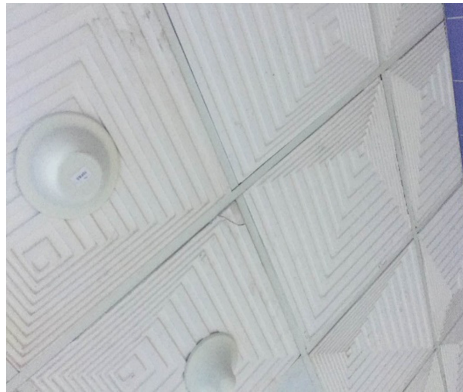
Fig. 3. DASs installed in the ceiling of the building indoors connected to the splitter.
